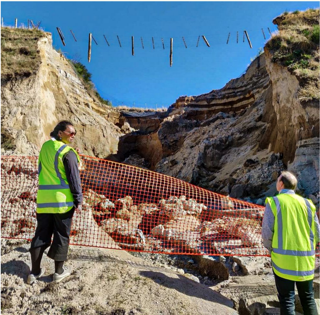
Figure 1: Spill site 05/03/2019 – Source: TMTB
